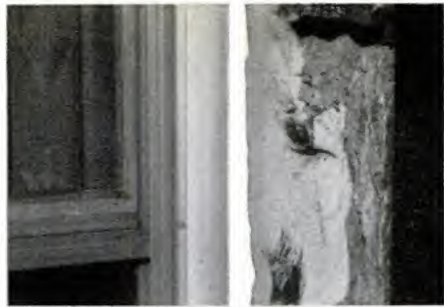
POOR CAULKING leaves end grain exposed. Moisture then creeps in between casing and masonry wall
